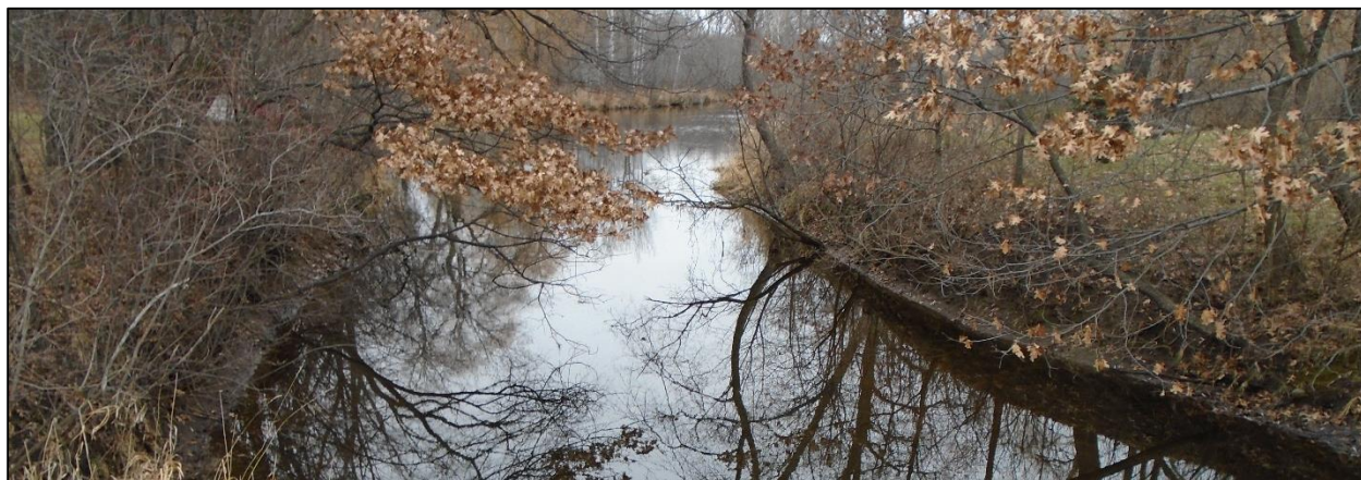
Figure 18. Proposed bank stabilization site, north of the E Pleasant Lake Rd bridge on the Deep-Pleasant channel
