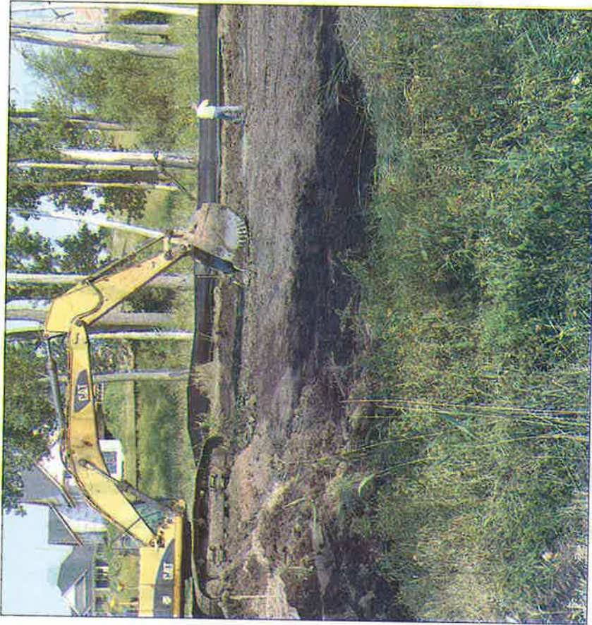
Excavation is being used to create wetland contours for water treatment and habitat improvements.
